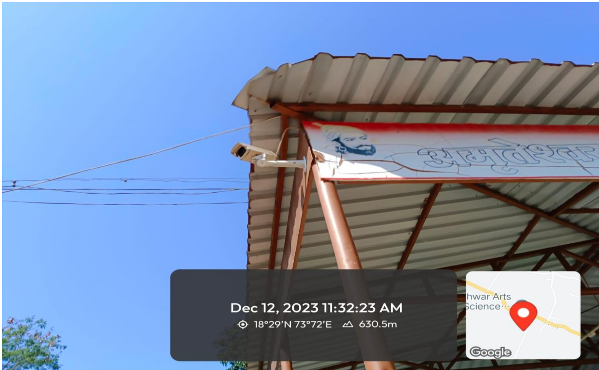
CCTV Camera at College corridor
