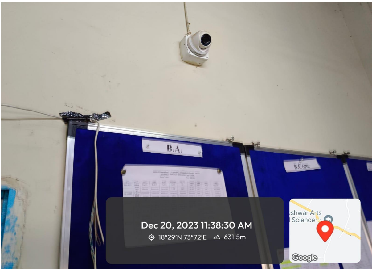
CCTV Camera at College Exam Room
