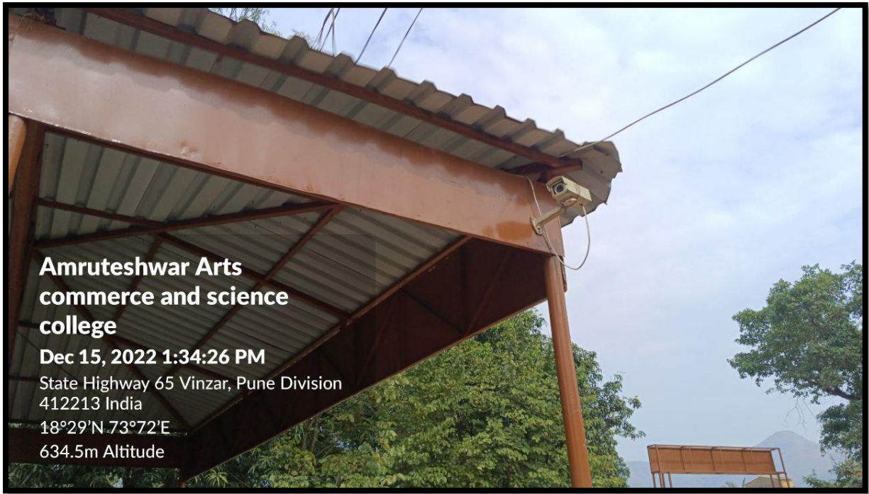
CCTV at College Campus
